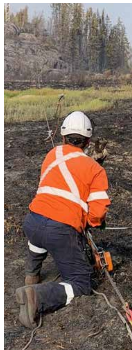
Wildfires under the transmission line from Taltson caused damage in the summer of 2022.
