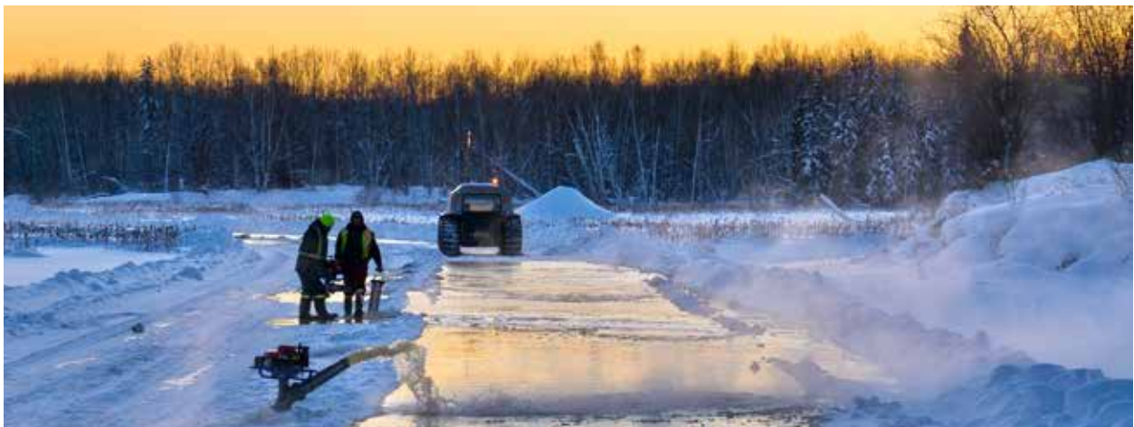
Construction of the Taltson Winter Road over the past several years was critical to transporting key components required for the unit overhaul.
