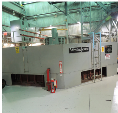
Main generating unit at Taltson
