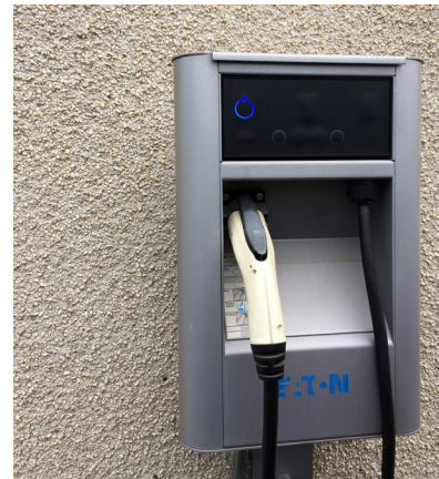
Electric Vehicle charging station at the AEA's Yellowknife office.
