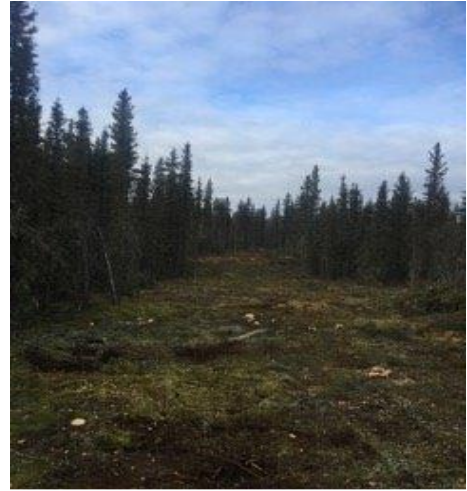
Construction proceeding on the Rae Extension Section of the Behchokò Access Trail.
