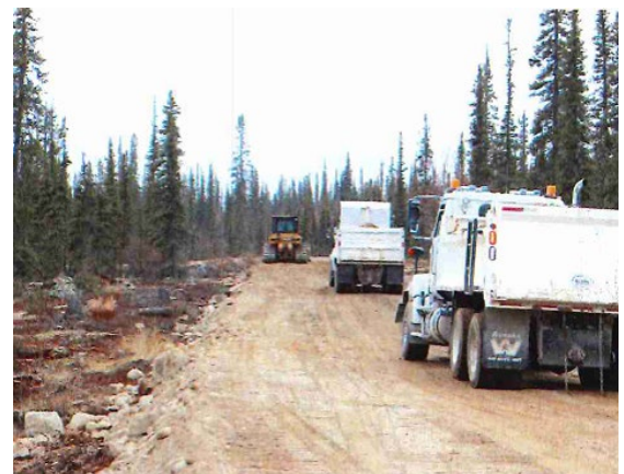
Bulldozer and dump trucks during summer 2020 construction on the Wekweètì Access Road.
