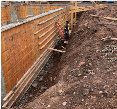
The foundation for a new diesel generating plant being installed in Łutselk'e. The new plant will have high efficiency generators and is located outside of the centre of the community, moving fuel storage away from Great Slave Lake as well as reducing noise and GHG emissions.
