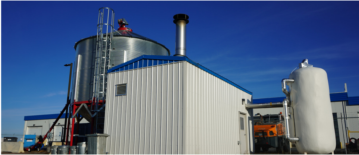
Wood pellet boiler at Yellowknife Airport's combined services building.
