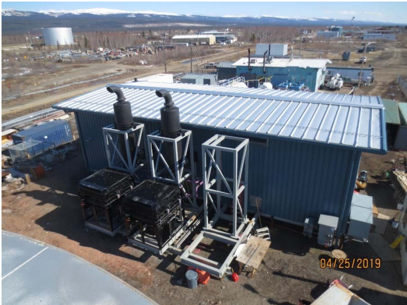
A new backup diesel plant in Norman Wells was commissioned in 2019-20
