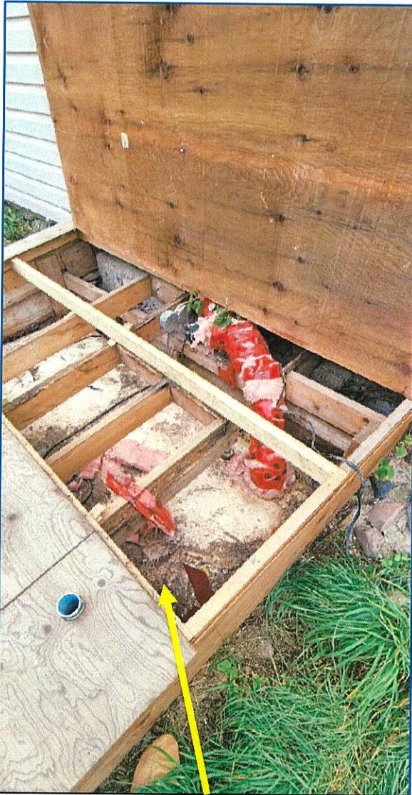
These 500 insulated tanks are over 45 years old and the heat trace stop working and the tank freezes year after year.
