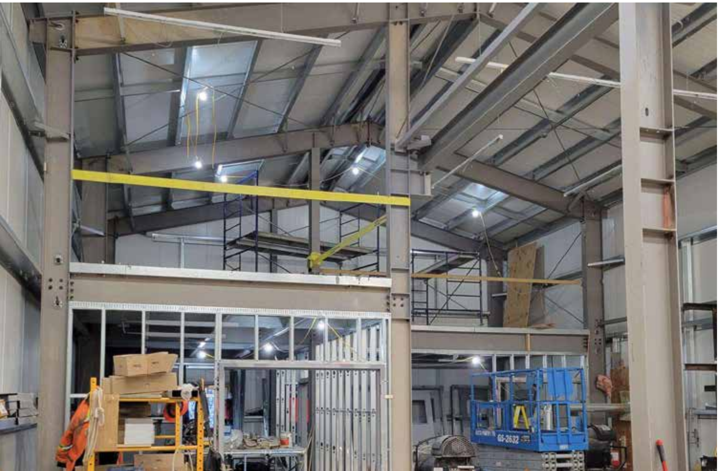
The interior of Łutselk'e's new diesel power plant. The new plant is scheduled to be operating by the end of the 2022-2023 fiscal year.
