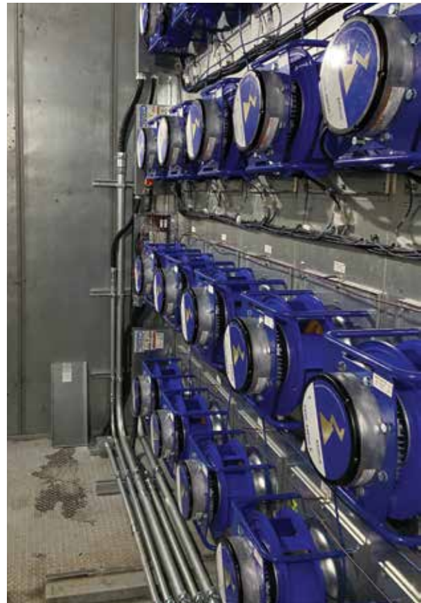
This modular fan wall reduces electricity consumption in Yellowknife's Laing Building.
