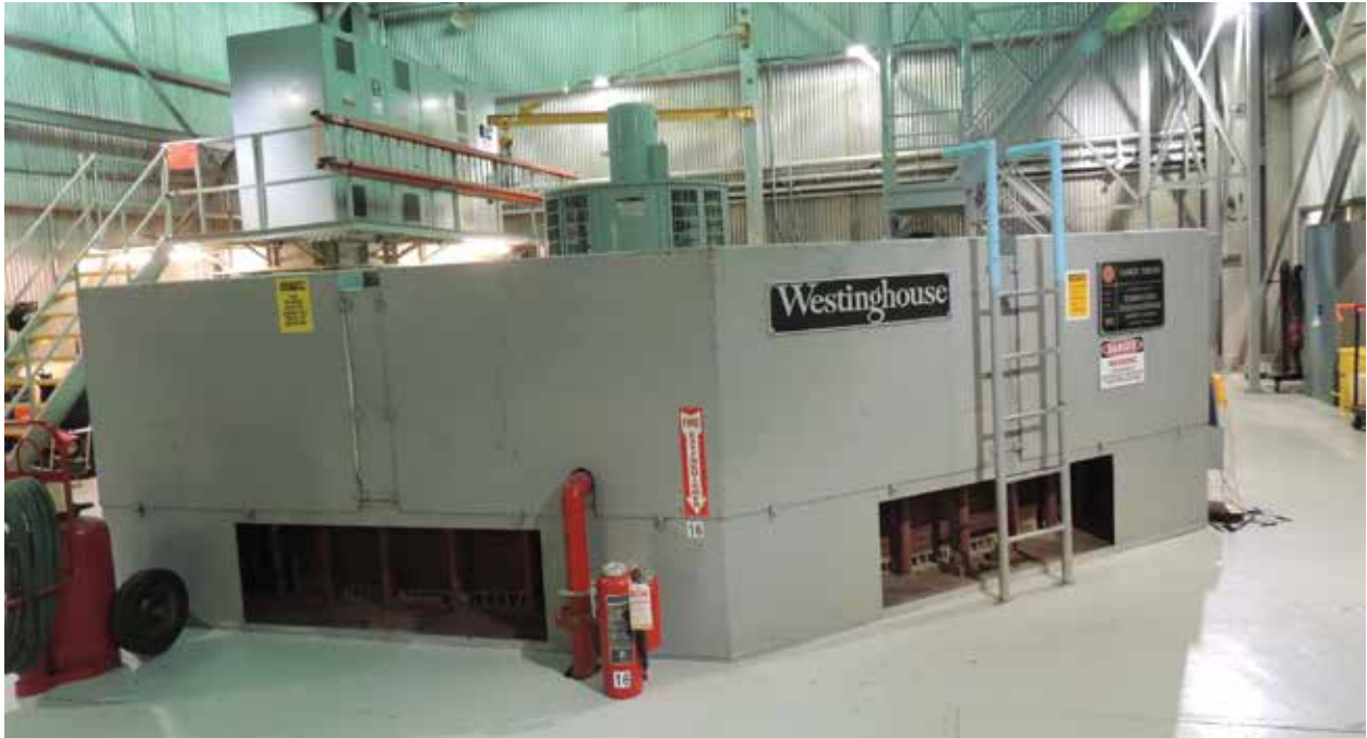
Current generation unit at the Taltson Hydro facility.
