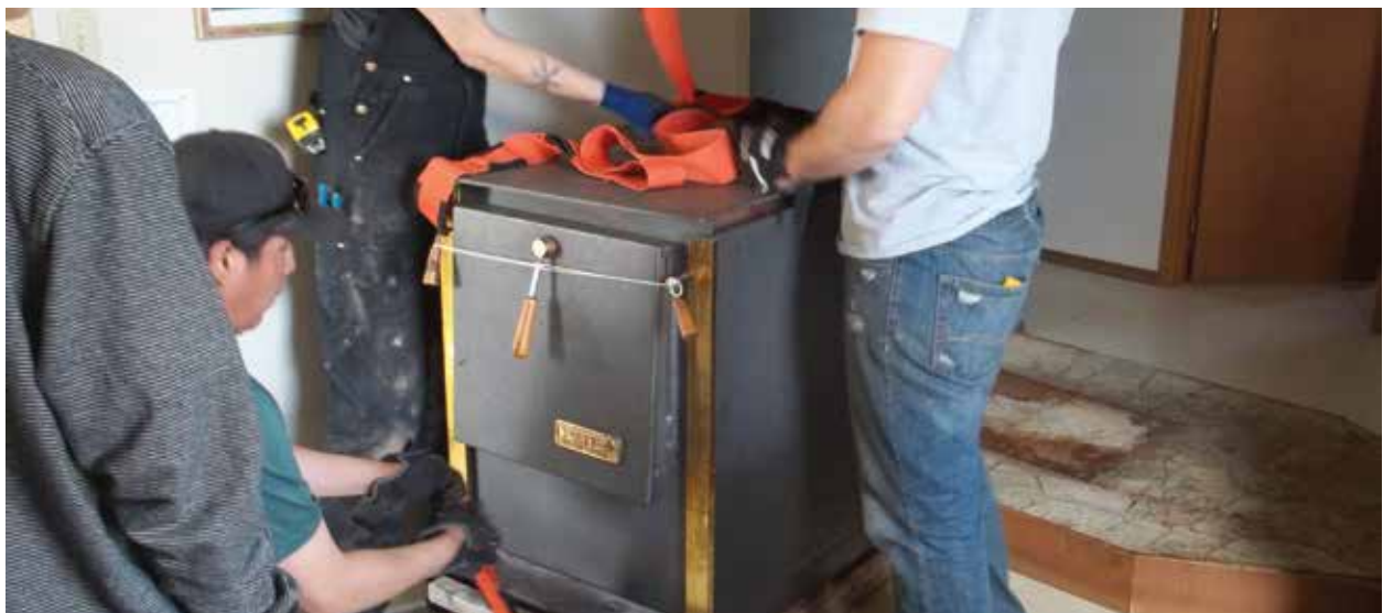
A project crew removes an old stove from a home as part of the AEA's community wood stove program.
