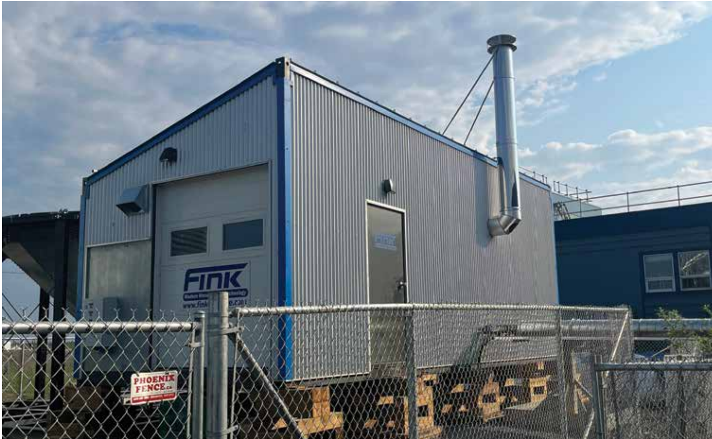
Wood Pellet Boiler Container at Moose Kerr School.
