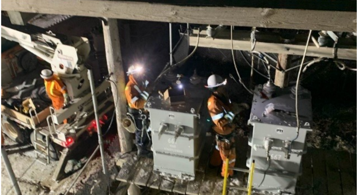
Our team responds to all problems, regardless of the time or weather conditions. In this photo, linepeople are replacing three feeder transformers in Tuyktoyaktuk. The salt air in coastal communities causes corrosion (rust) to occur more quickly than in other locations.
