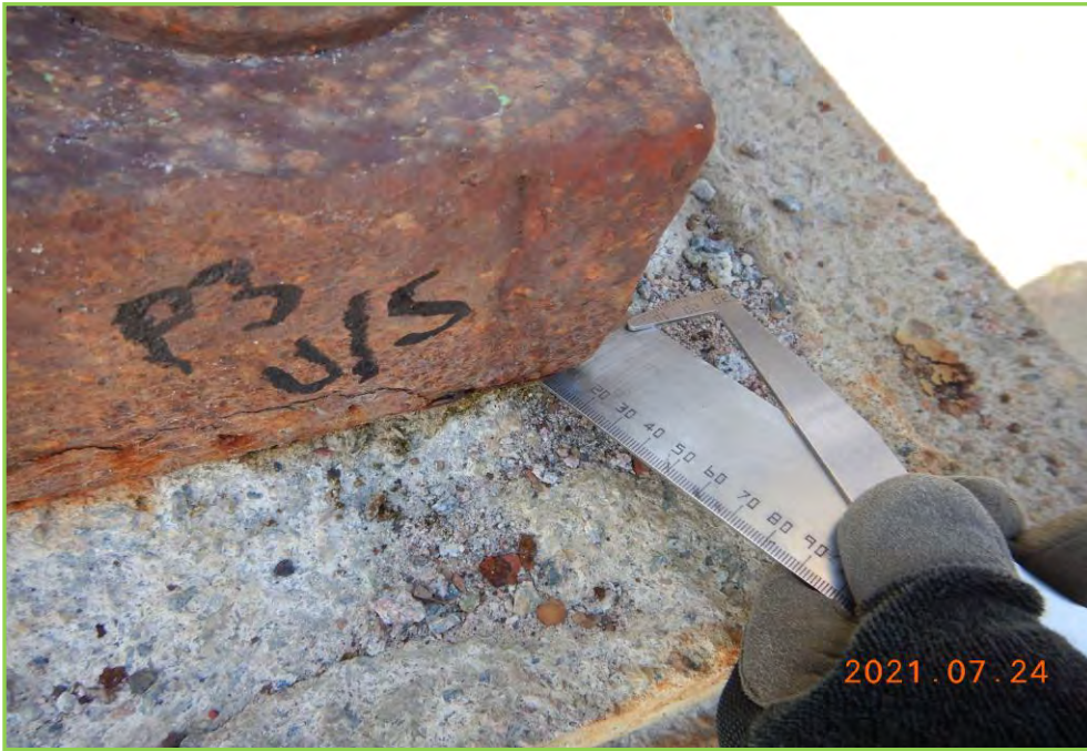
Photo 061 – Concrete/Grout spall at Bearing Seat, Pier 3, US
