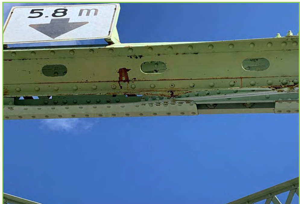
Photo 084 – Span 1 Portal, Minor Deformed on the Bracing Due to High Load Damage
