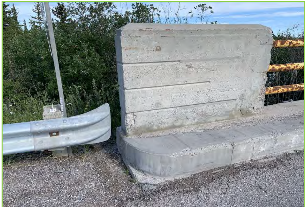
Photo 080 – Guardrail at Abutment 1, Northwest, No Connection to Concrete Barrier
