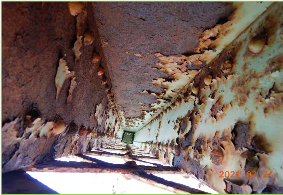
Photo 097 – Vertical at Span 1, Looking inside. Typical Light Corrosion and Minor Section Loss at Splash Zone
