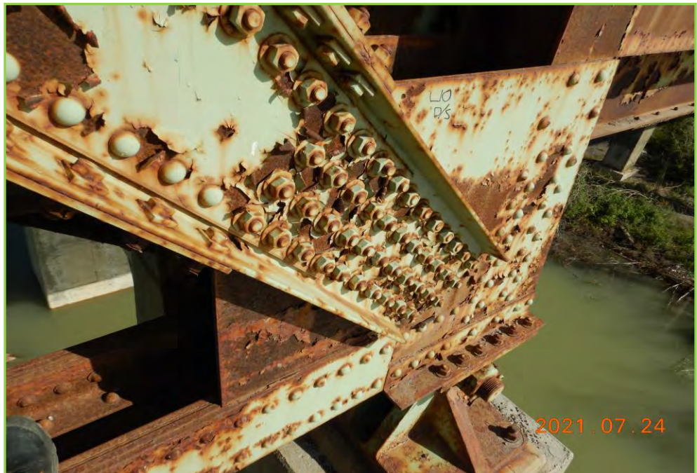
Photo 096 – Truss Connections at Pier 1, Span 1, Light Corrosion with Minor Section Loss
