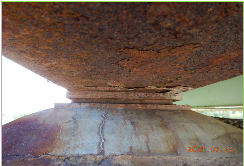
Photo 052 – Girder 1 at US, Pier 2. Bottom Flange, Light Corrosion with Section Loss 0-5%.
