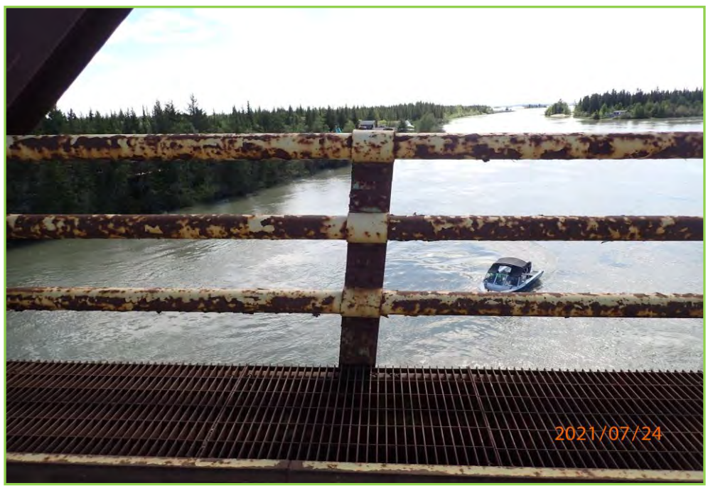
Photo 032 – Handrail Post at Span 4, 4th form Abutment 1 at Southside (DS), Slightly Rotated to the West. Light Corrosion with Paint Peeled
