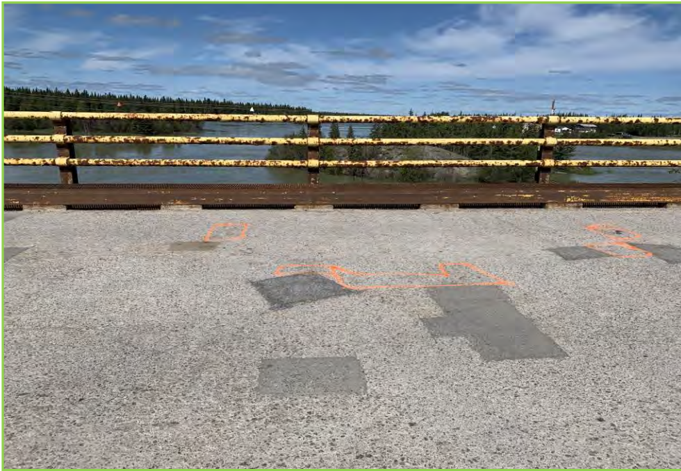
Photo 033 – Handrails at Span 2, Typical paint peeled, Light Corrosion with No Section Loss
