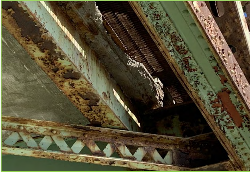
Photo 19 – Deck Soffit- Exterior, Severe Spall with Rebar Exposed (Typical)
