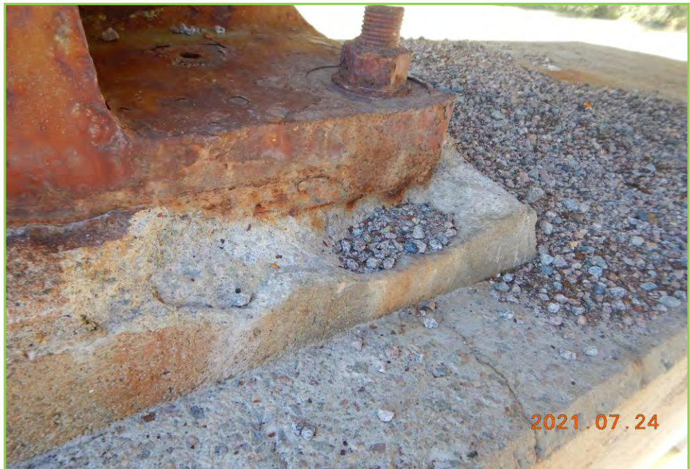
Photo 060 – Concrete Scaling and minor Spall on the Bearing Seat, Pier 3
