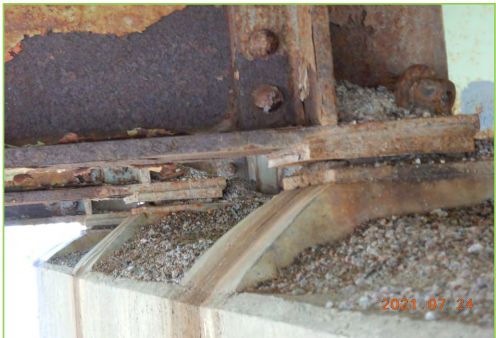
Photo 056 – Anchor Bolt Shear Off at Interior Girder (G3), Span 2
