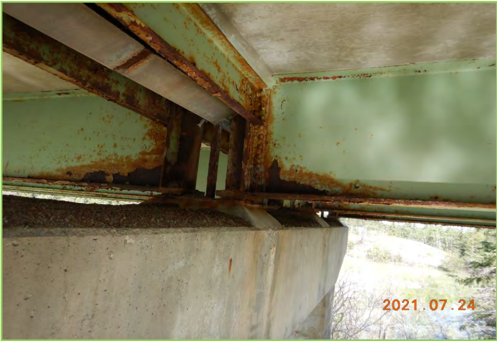
Photo 054 – Top of Pier Cap, Pier 4. Light Corrosion at the End Diaphragm.
