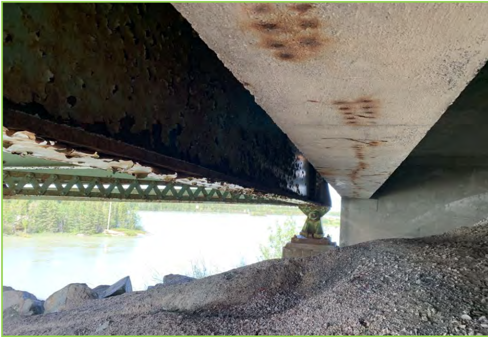
Photo 079 – Bottom of Ballast Wall at Abutment 2, Staining due to Rebar Corrosion with not Enough Cover
