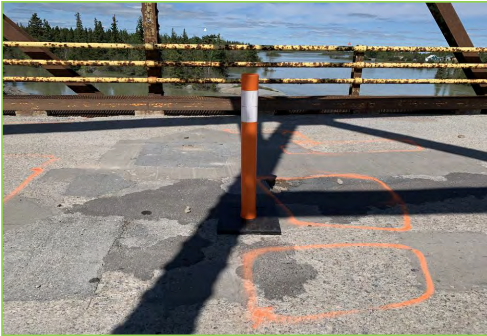
Photo 15 – Delamination of Concrete Deck at Span 4 (Typical)
