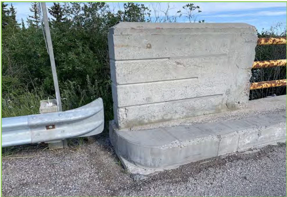
Photo 9 – Concrete Parapet and Curb at Abut 1, Wide Cracks and Minor Spall noticed
