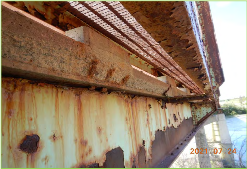
Photo 067 – Exterior Girder (G4) at Span 3, US, Light Corrosion with Minor Section Loss
