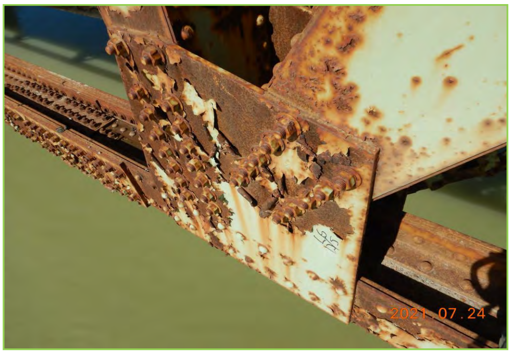
Photo 094 – Truss Connections at Span 4, Typical Light Corrosion with Minor Section Loss
