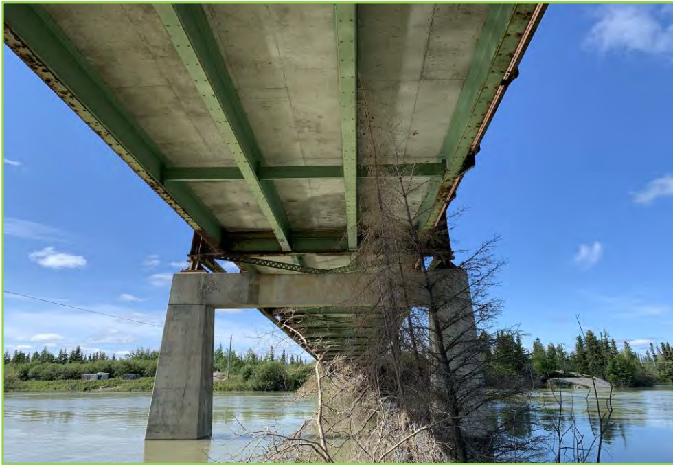
Photo 043 – Underside of Span 2, Looking Pier 1, Girders, Typical Light Corrosion at the Bottom Flange of the Exterior Girders.
