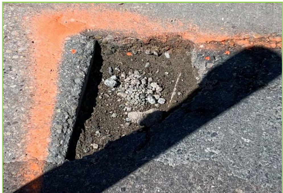
Photo 16 – Concrete Spall (Pothole) at Span 1
