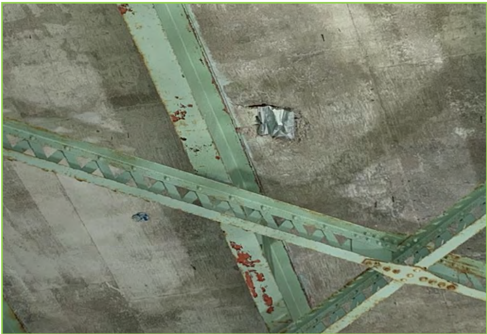
Photo 023 – Deck Soffit Full Depth Patching at Span 2
