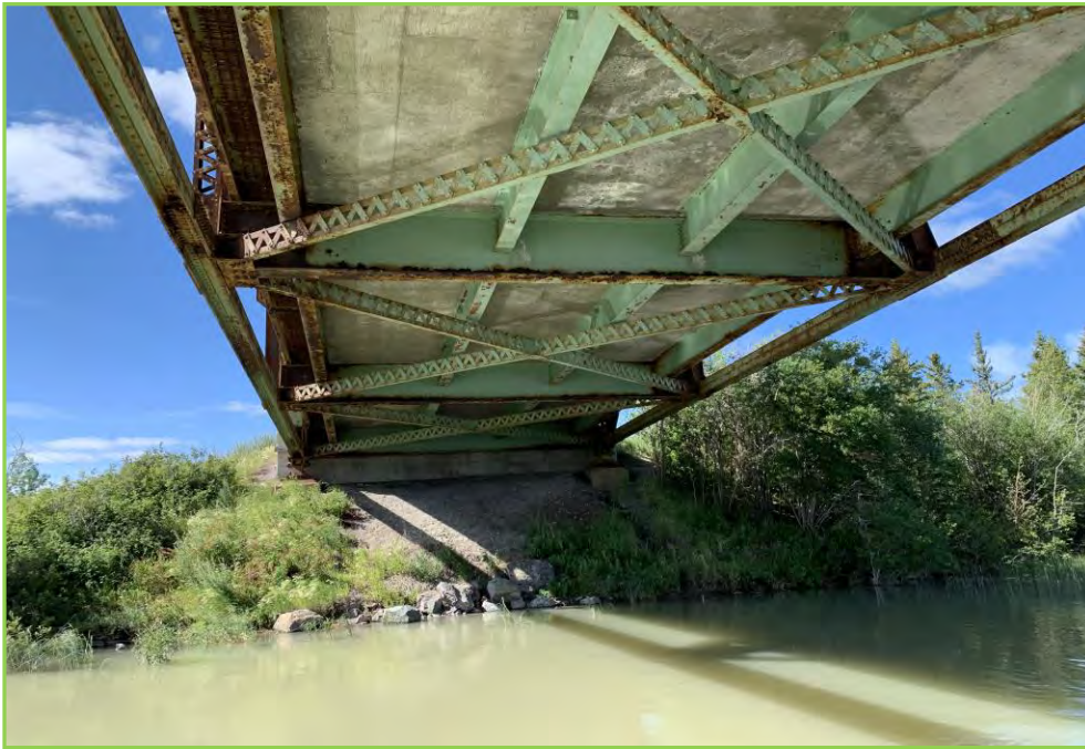
Photo 041 – Underside of Span 1, Looking Abutment 1, Stringers and lateral Bracings, Typical Light Corrosion at the Bottom Flange of the Floor Beams and Exterior Stringers.
