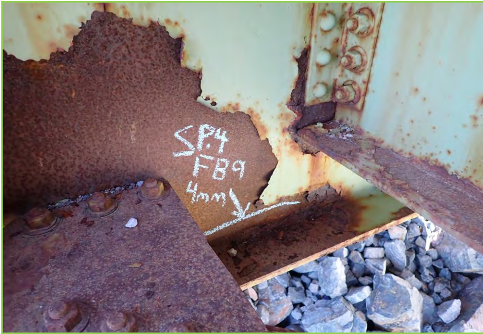
Photo 037 – Intermediate Floor Beam at Span 4, 9 th bay, 4mm Section Loss on the web Near Bottom Flange
