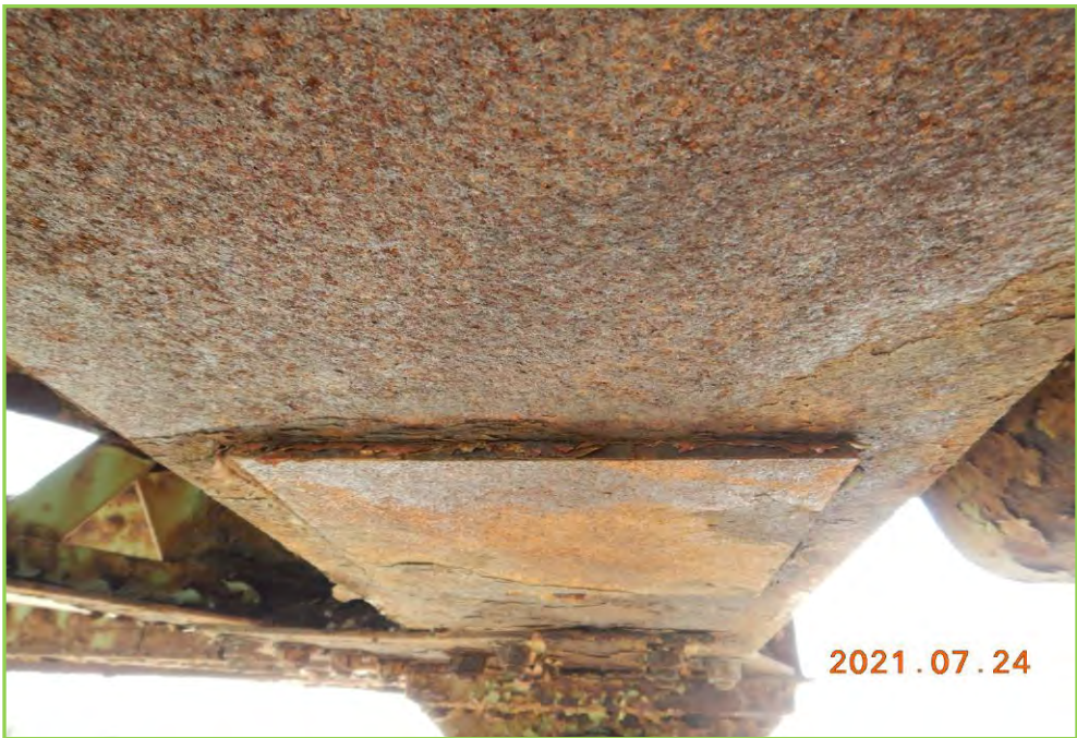
Photo 065 – Girder End of Exterior Girder at Span 3, Light Corrosion with Minor Section Loss
