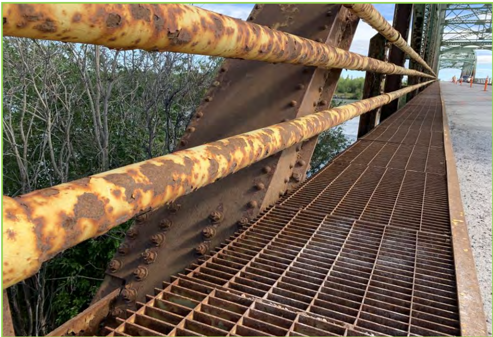
Photo 031 – Steel Grating/Curb and Handrails at Span 1, light Corrosion, Rusting with Coating Failed
