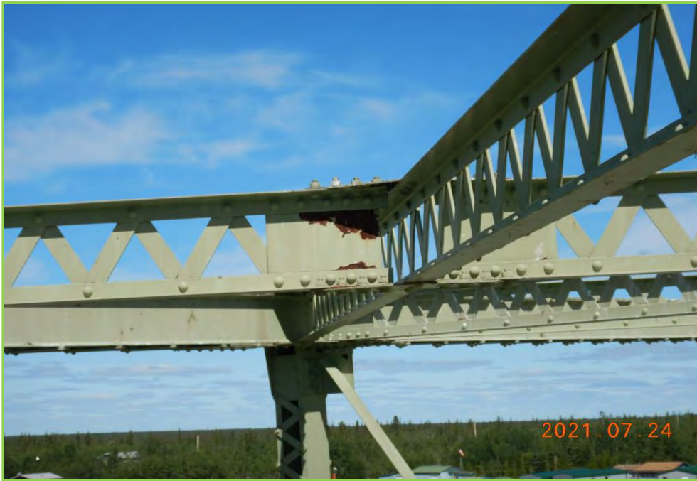
Photo 083 – Span 1, Truss Element, Light Corrosion at the Connection of Sway Bracings
