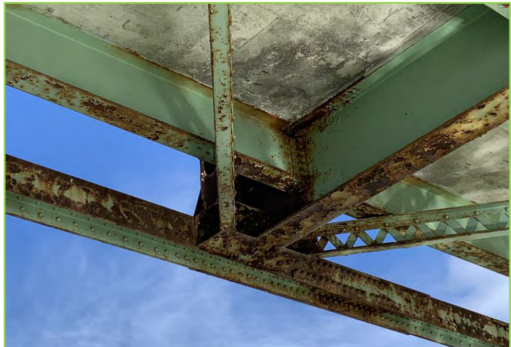
Photo 020 – Deck Soffit at Span 1 7 th Intermedia Floor Beam, US,
