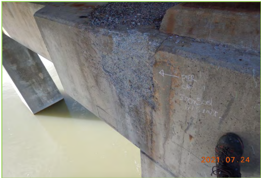
Photo 046 – Concrete Spall at Pier 1 Cap, 300mm x500mm.
