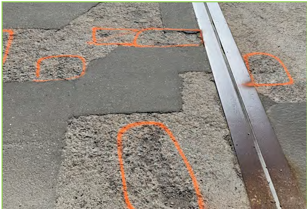
Photo 028 – Deck Joint at Pier 3
