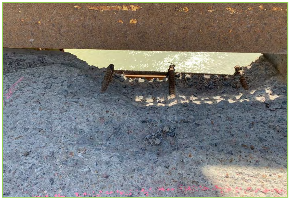
Photo 18- Deck top Severe Spall with Rebar Exposed (Typical)
