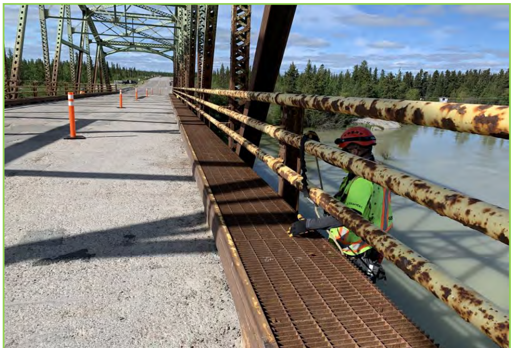
Photo 030 – Steel Grating/Curb at Span 1, light Corrosion, Rusting with Coating Failed
