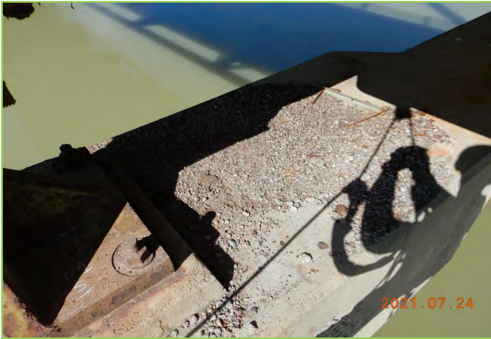
Photo 049 – Gravel on the Pier Cap, Pier 1
