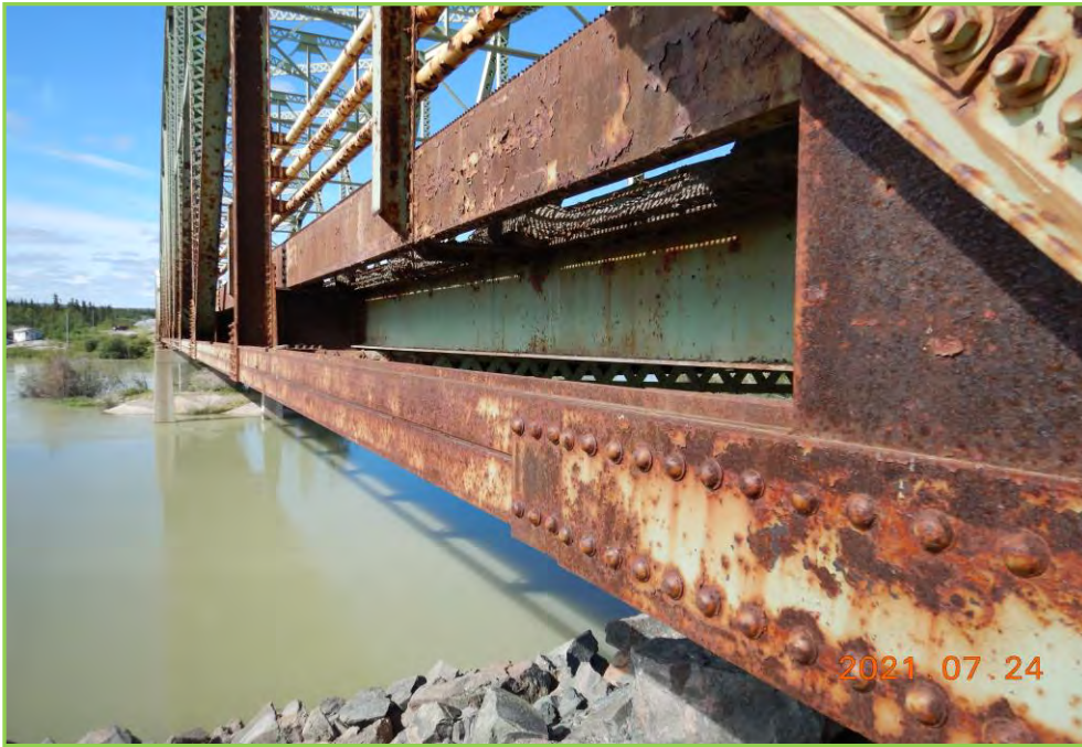
Photo 091 – Bottom Chord at Span 4, DS. Light Corrosion with Minor Section Loss
