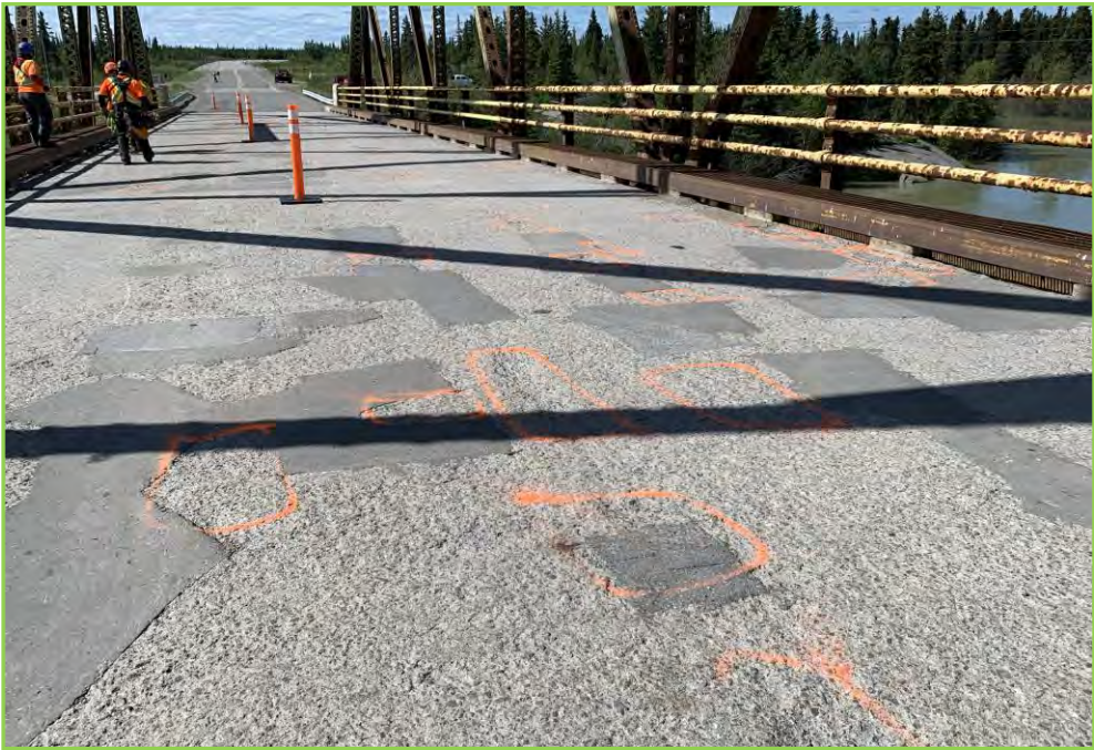
Photo 14 – Delamination of Concrete Deck at Span 4 (Typical)
