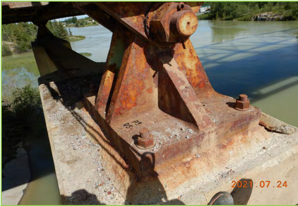
Photo 059– Rock Bearing at Pier 3, Light Corrosion
