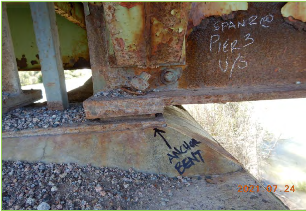
Photo 051 – Anchor Bolt Bent on the Span 2 of Girder 3, US, Pier 2
