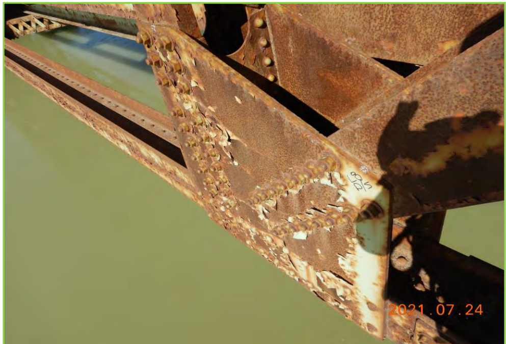
Photo 098 – Truss Connections at Span 1, Light Corrosion with Minor Section Loss
