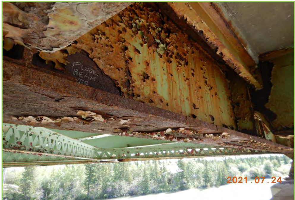
Photo 064 – Floor Beam L1 of Span 4 at Pier 3, Pack Rusting, Light Corrosion with Minor Section Loss
