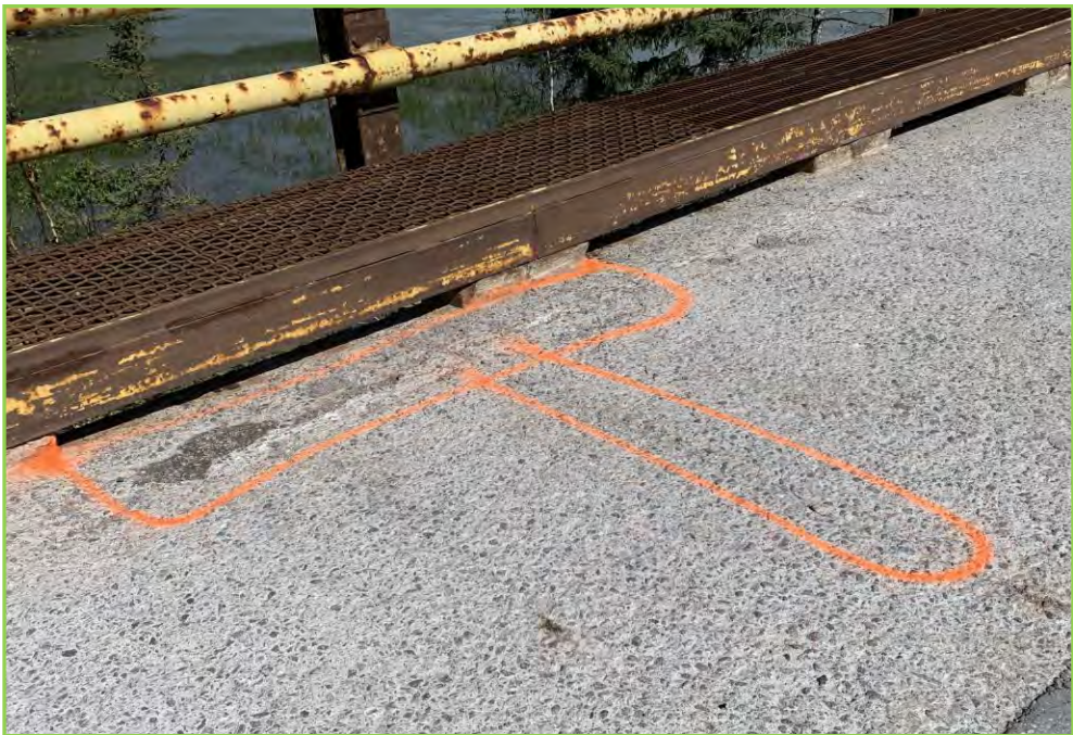
Photo 17- Wide Crack and Concrete Spall at Span 1
