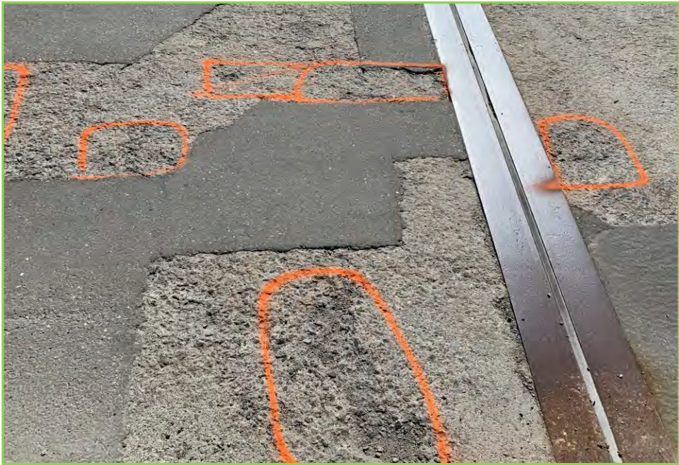
Photo 13 – Concrete Spall, severe scaling and delamination near Pier 3
