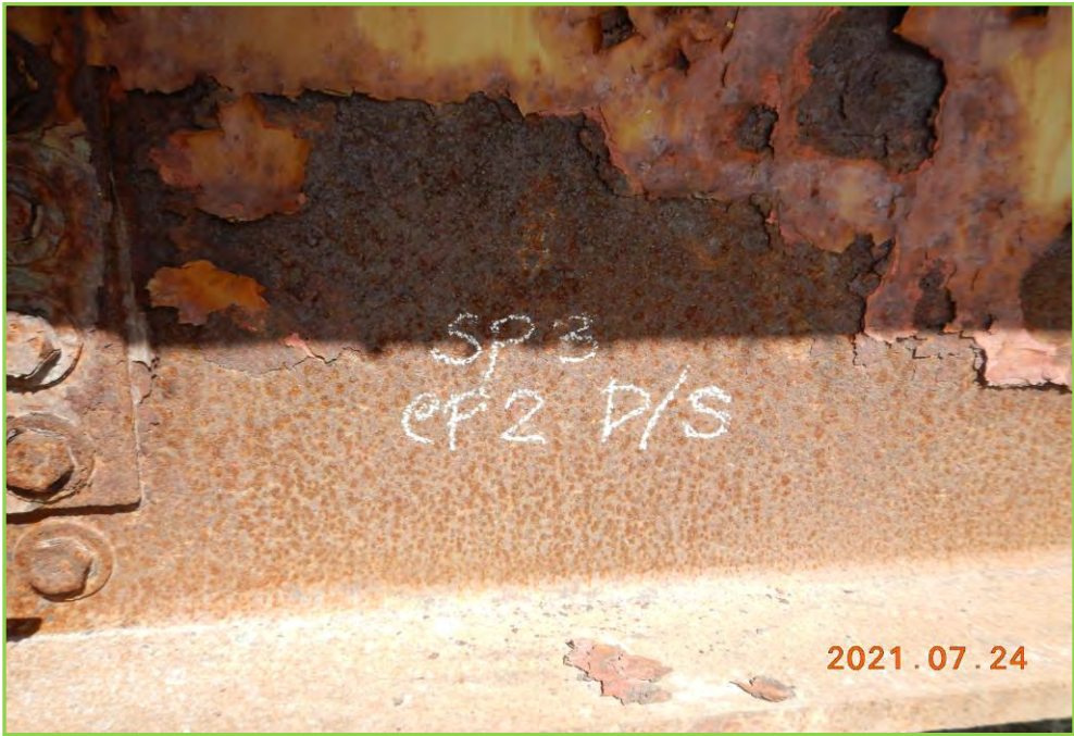
Photo 053 – Girder 4 at DS, Pier 2, Web, Light Corrosion with Section Loss 0- 5%.
