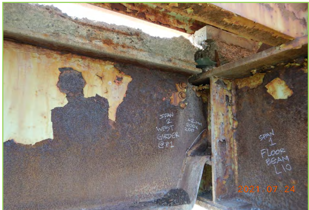
Photo 062 – Span2 , West Exterior Girder Support on Floor Beam L10 of Span1, Light Corrosion, Minor Section Loss, 200x200mm, 2 mm
