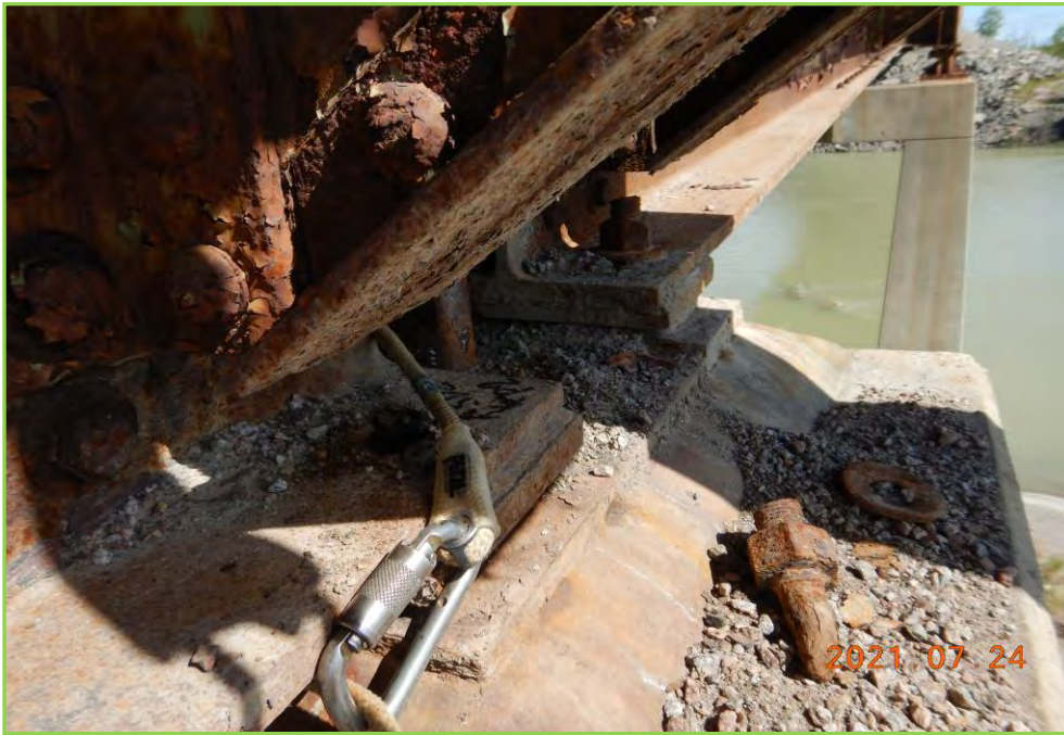
Photo 055 – Anchor Bolt Shear Off at Exterior Girder(G4), Span 2
