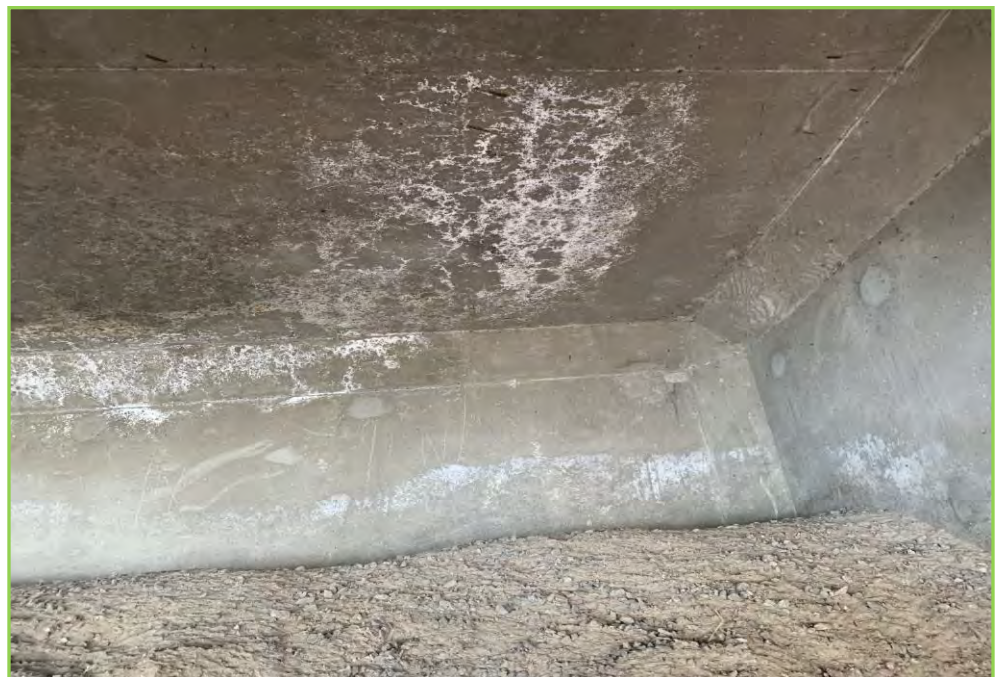
Photo 064 – Light Scale and Efflorescence on Roof Slab
