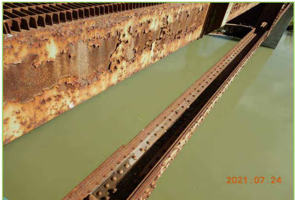
Photo 092 – Bottom Chord at Span 1, DS. Light Corrosion with Minor Section Loss
