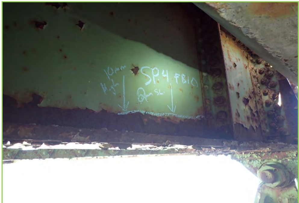
Photo 038 – Floor Beam at Span4, L10, Pack Rusting Along Bottom of Web, Just Above Bottom Flange with 2 mm Section Loss.
