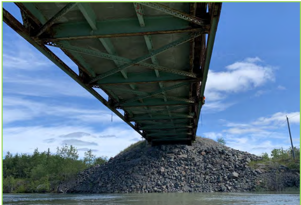
Photo 042 – Underside of Span 4, Looking Abutment 2, Stringers and Lateral Bracings, Typical Light Corrosion at the Bottom Flange of the Floor Beams and Exterior Stringers.
