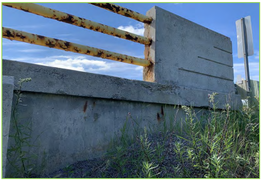
Photo 10- Concrete Parapet and Wingwall at Abut 1, North, Severe Scaling and Minor Spall
