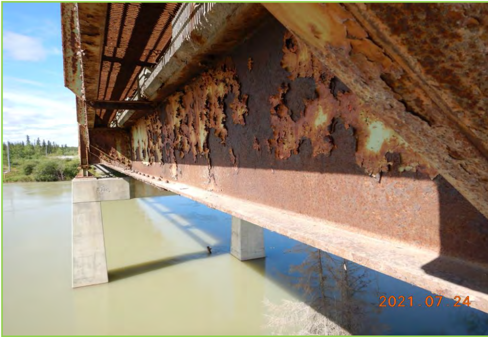
Photo 063 – Typical Exterior Girder at Span 2, Light Corrosion with Minor Section Loss
