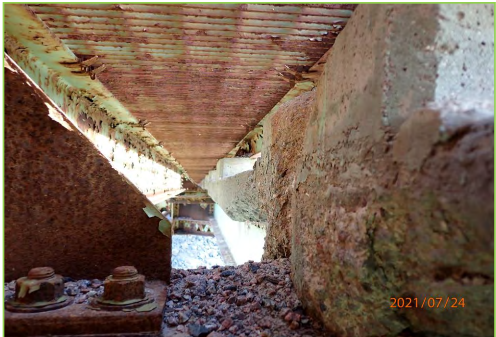
Photo 034 – Underside of Concrete curb /Steel Grating, Light Corrosion.
