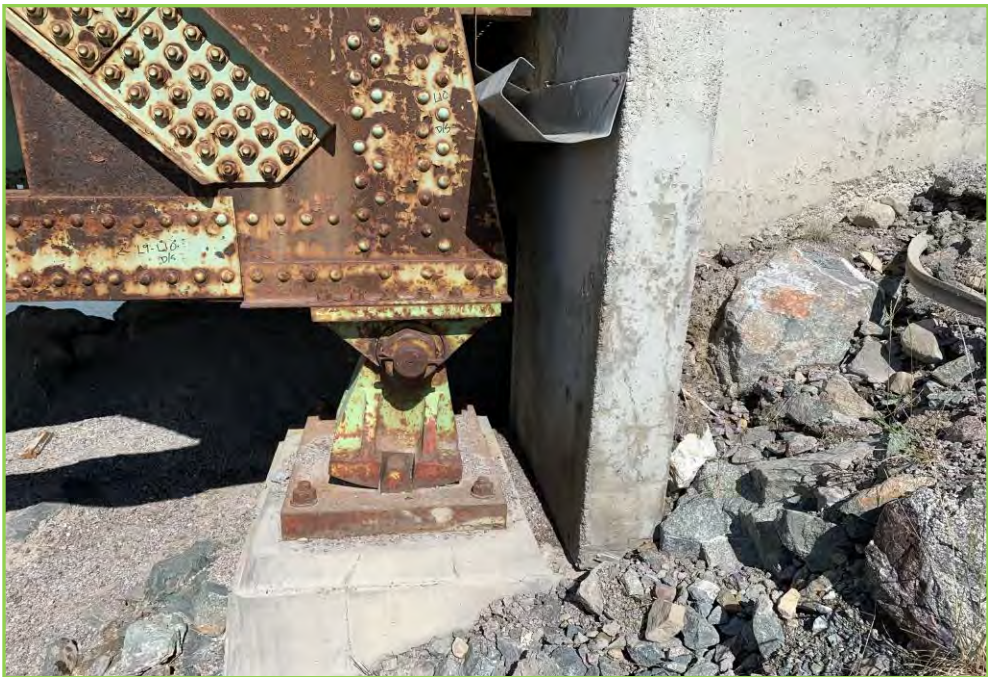
Photo 075 – Rock Bearing at Southeast, Light Corrosion
