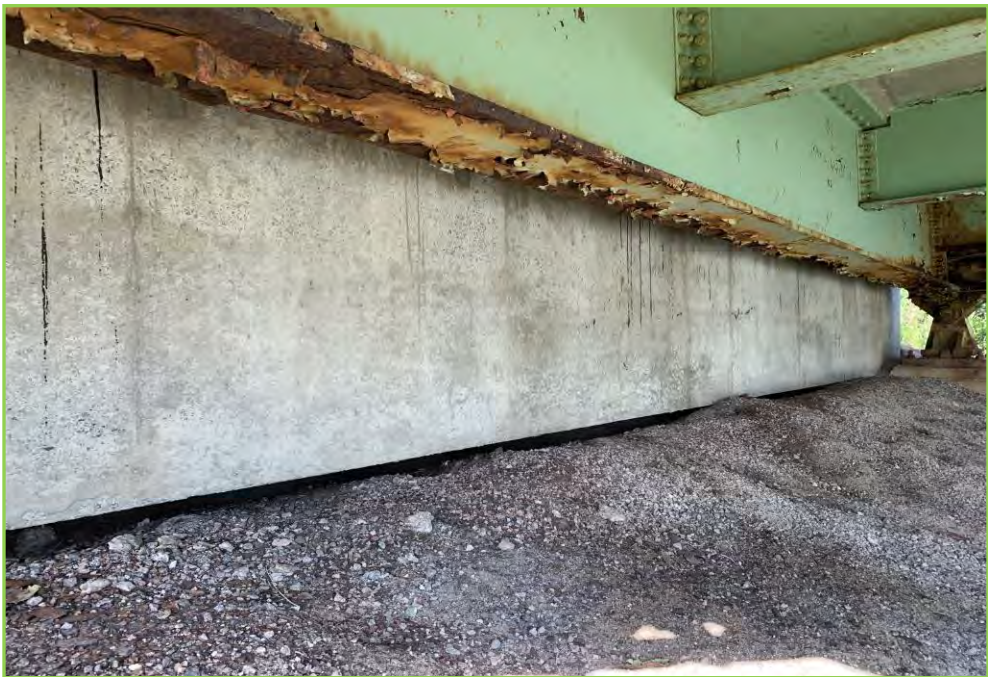
Photo 3 – Abutment Wall at Abut1, Headslope Settled
