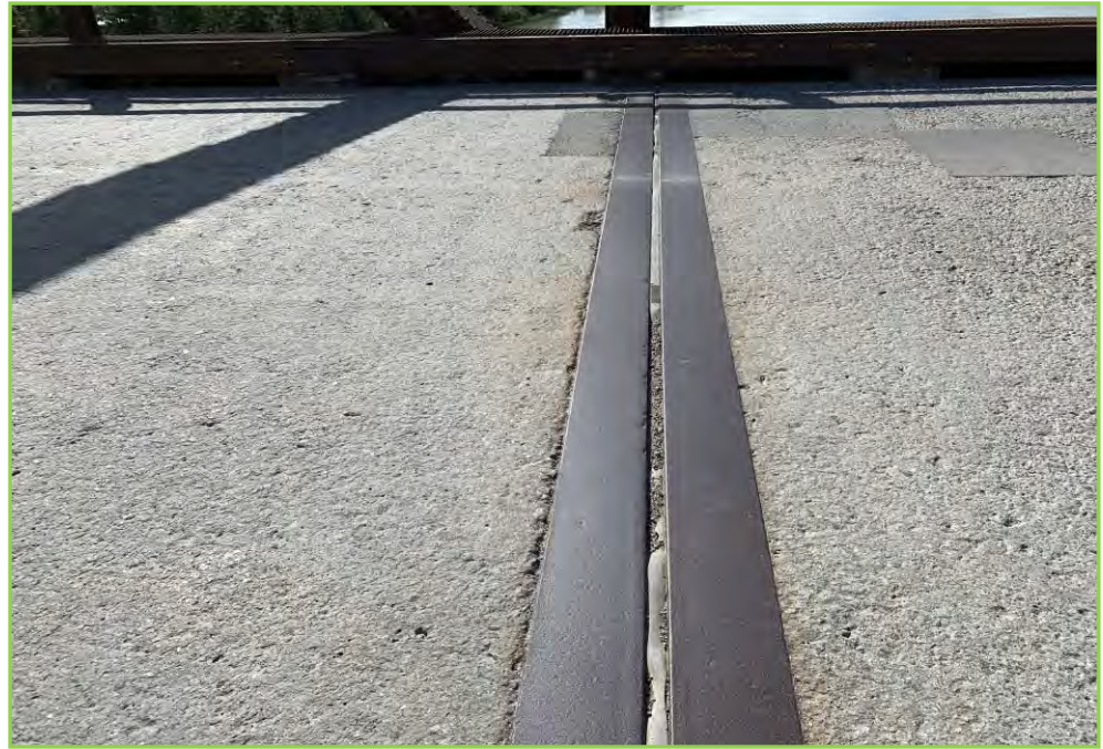
Photo 026 – Deck Joint at Pier 1
