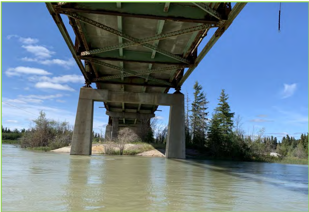
Photo 057 – Pier 3 Looking West, In General Fair Condition
