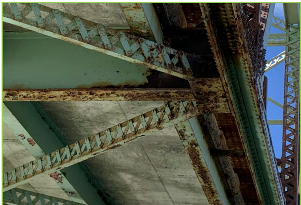
Photo 044 – Connection of Floor Beam, Lateral Bracing and Bottom, Light Corrosion with Minor Section Loss
