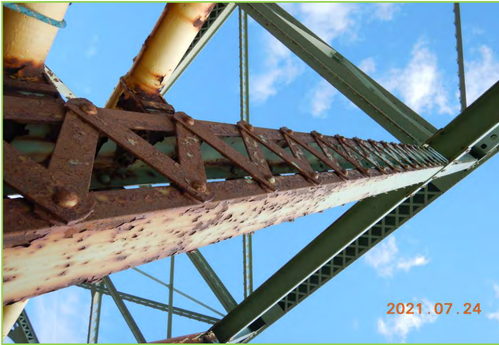
Photo 095 – Vertical at Span 4, Typical Light Corrosion and Minor Section Loss at Splash Zone
