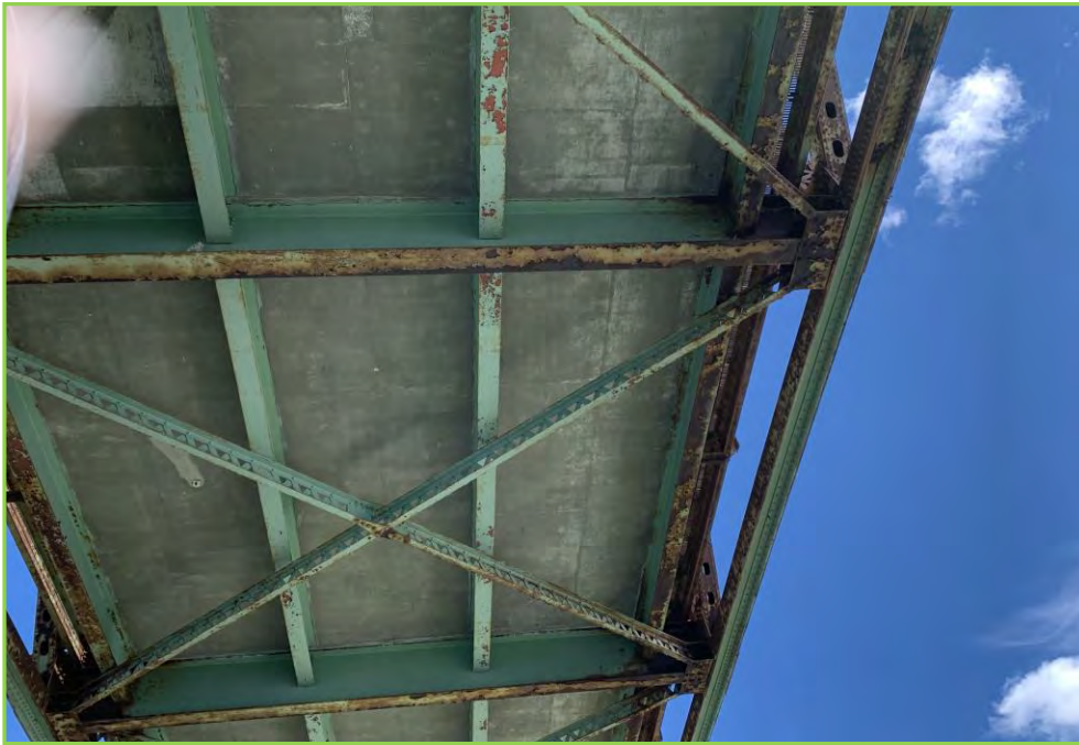
Photo 021 – Deck Soffit at Span 1 (typical)
