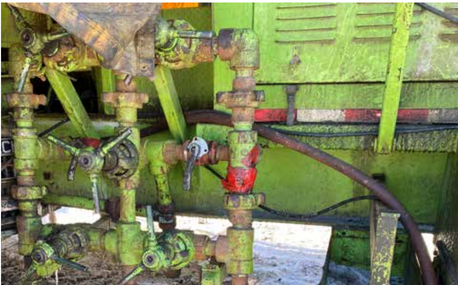
Manifold, Cameron Hills, March 2023. (Credit: OROGO)
