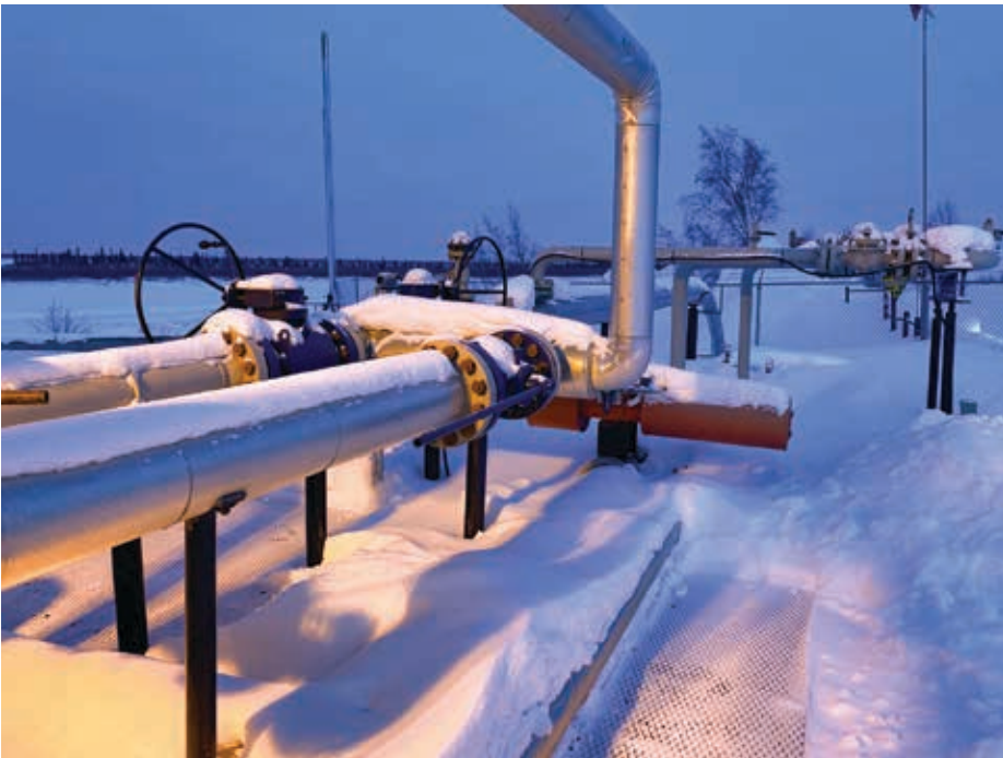
Gate station, Ikhill Gas Project, Inuvik, March 2024. (OROGO)
